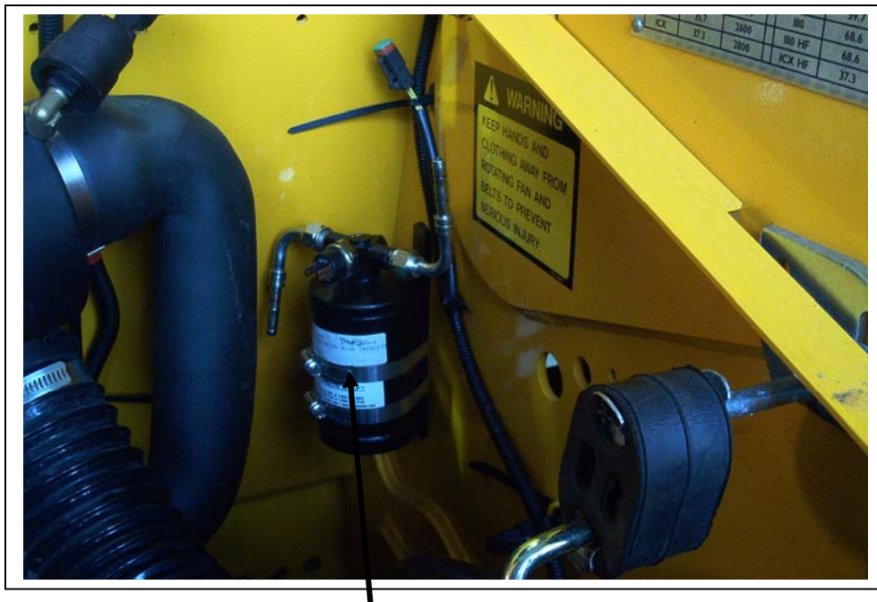
Drier installed and secured with gear clamps
