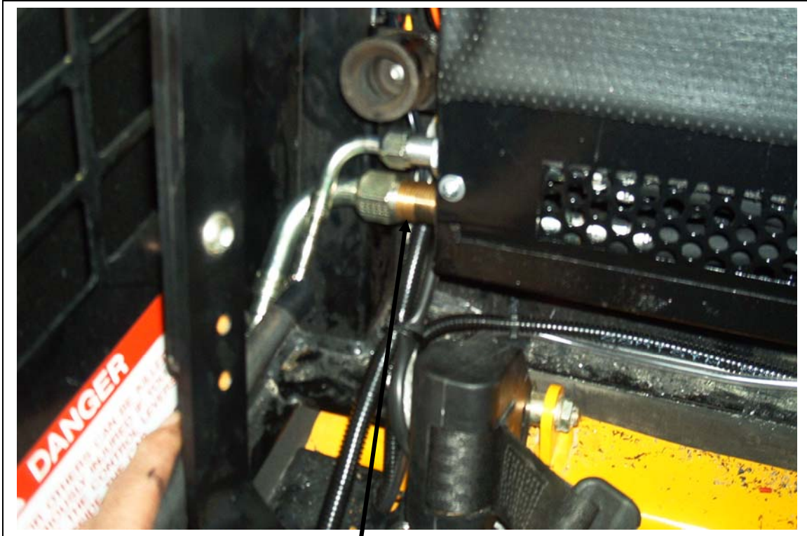
Hose fittings connected to evaporator box.
